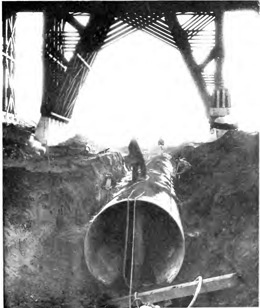
Top—Picture of Rindler Creek bridge in American Canyon to be replaced by fill and below, large metal culvert being placed to carry creek waters through fill.
